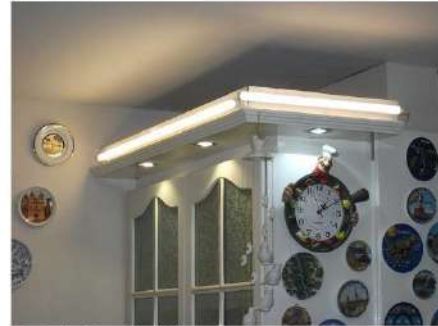
B: Kitchen lighting
